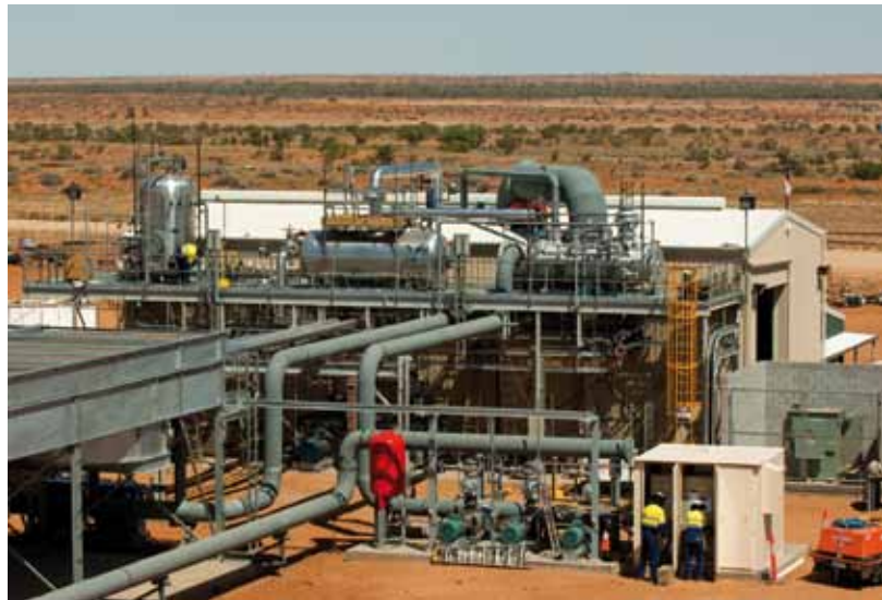
Power plant components behind the turbine hall and Visitors Centre
