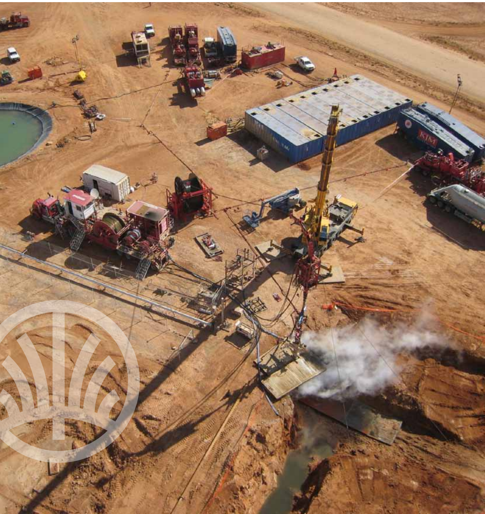
Habanero 3 well control incident during May 2009
