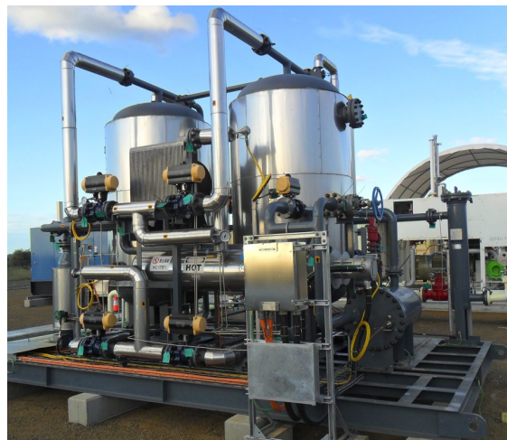
Figure 3: Commissioned dehydrator package, capable of reducing moisture content to less than 35mg/sm 3
