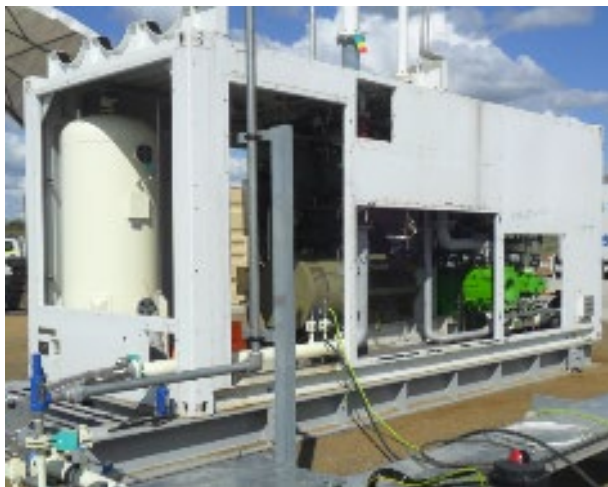
Figure 2: Commissioned modular compressor package, capable of compressing up to 1.7TJ of natural gas per day
