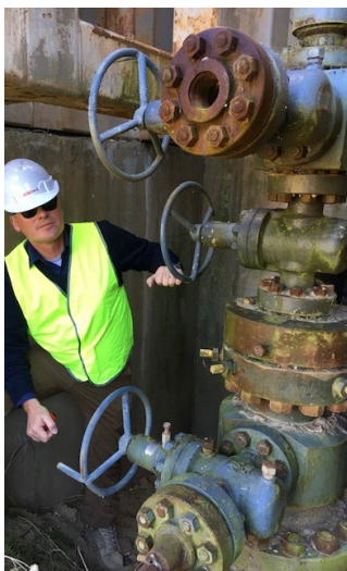
Established wellhead infrastructure at PL231 Reid's Dome.
