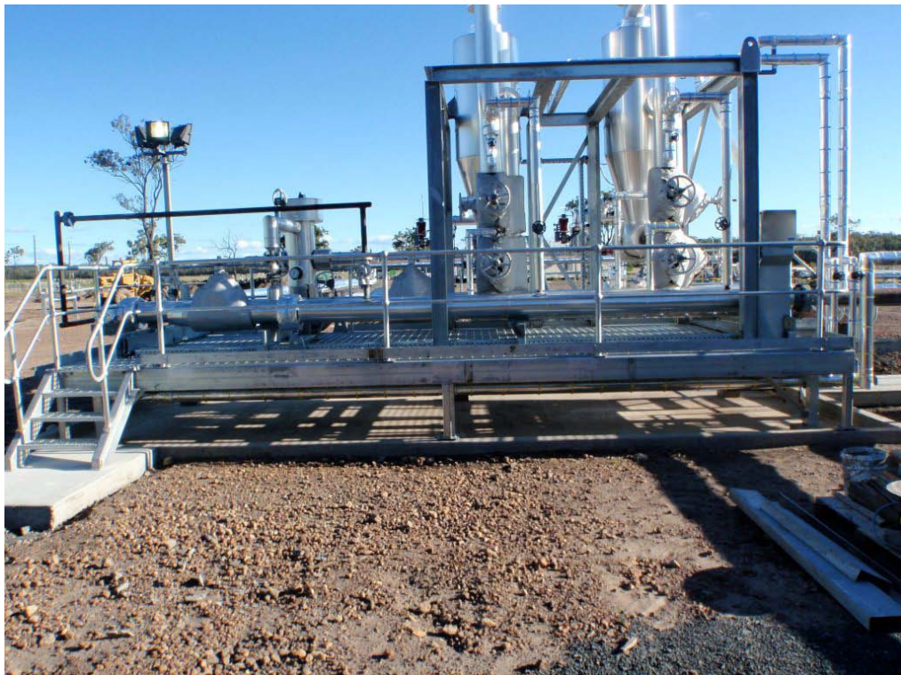
Panel 2 Knock out pots and access platforms
