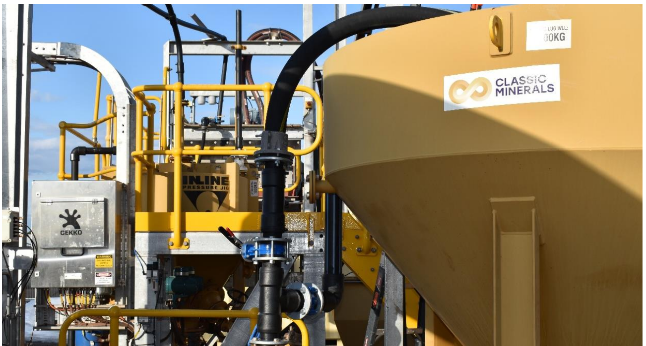
Figure 1: Gekko plant in Perth (part).
