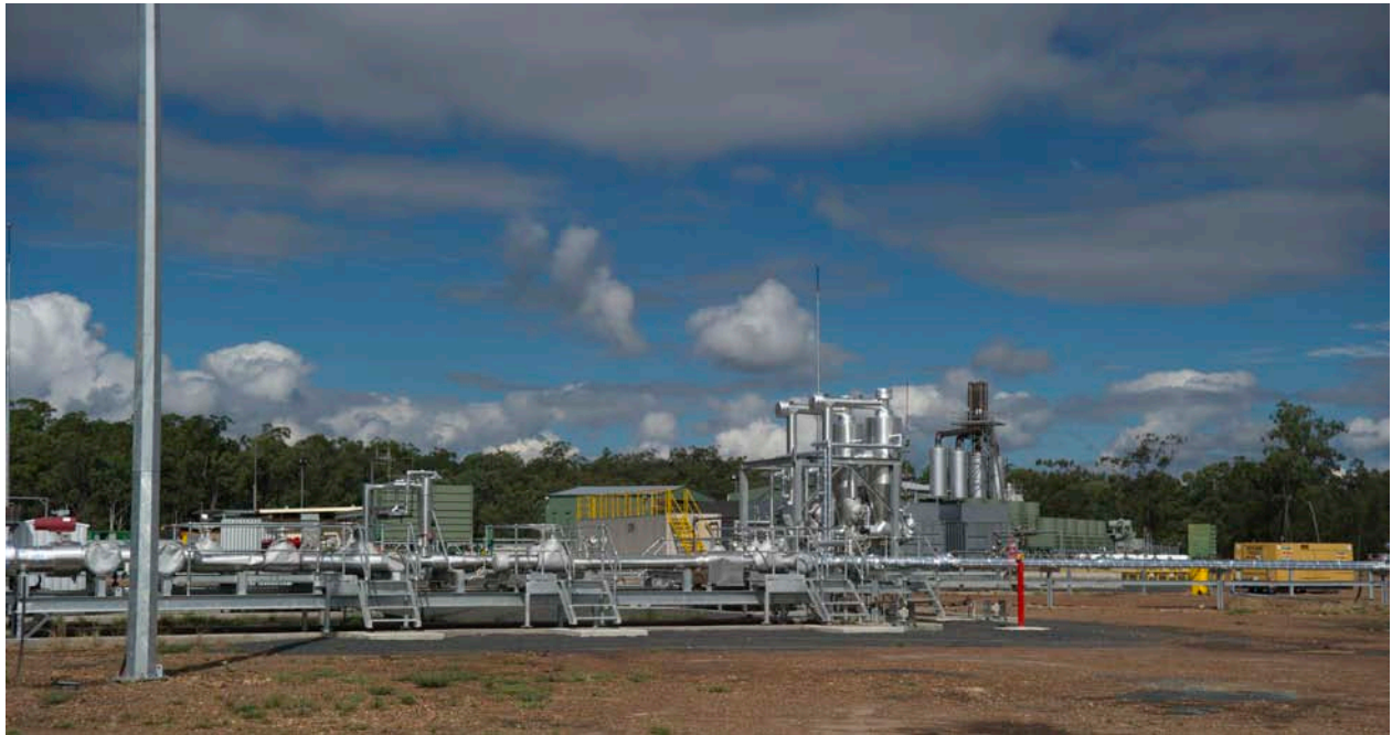
Gas Processing and gas delivery plant from panel 2 to 5MW Power Station May 2011 (power station rear right)
