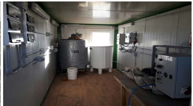
Pilot Plant Switchboards Room
