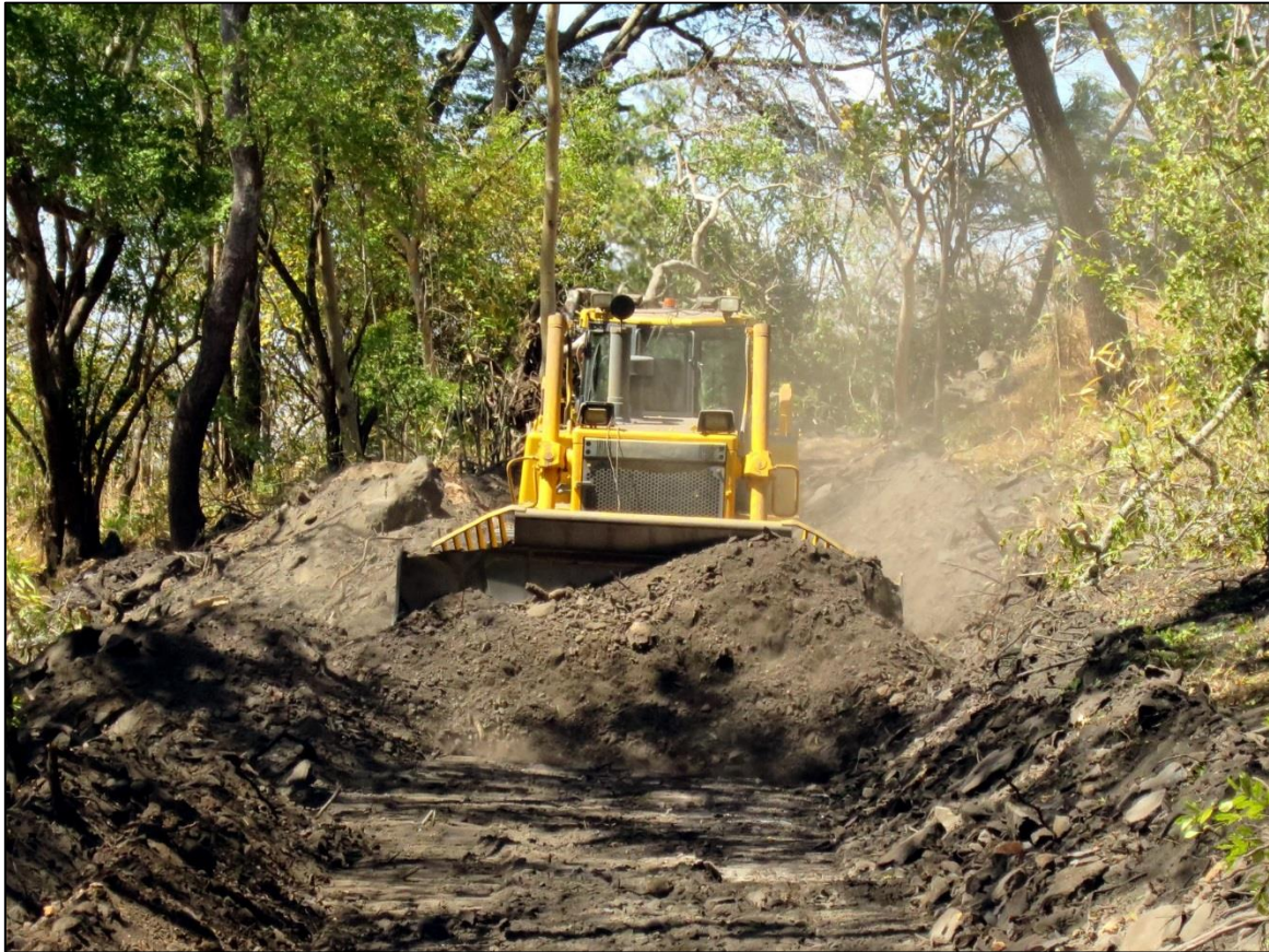
Figure 2. Excavation of Costean_N4 showing graphitic mineralisation at surface. Bulldozer is at approximately 6240E which is the eastern (footwall) contact of the Mutola Zone.
