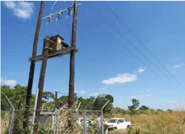
Figure 5 – Installed power lines and transformers
