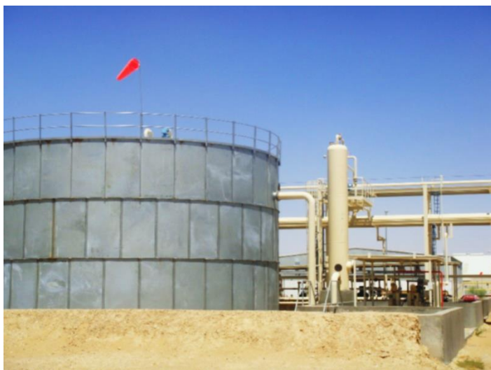
Damis (Block S-1) Production Licence – An Nagyah Oilfield production and storage facilities
