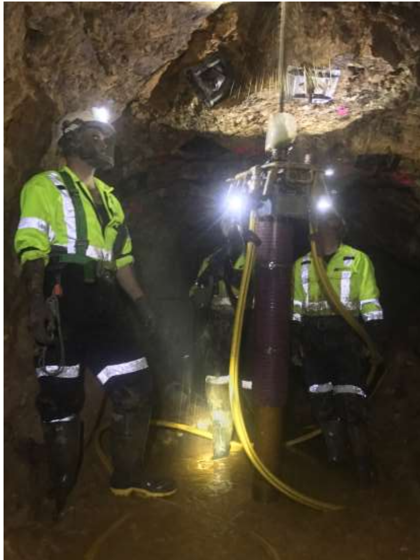
Figure 1 - Miners using a compressed air powered gopher to install rockbolts in the hangingwall of the No 8 level Drive
