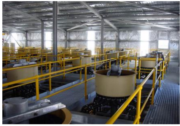
Figure 3: Distributors on upper floor of WCP
