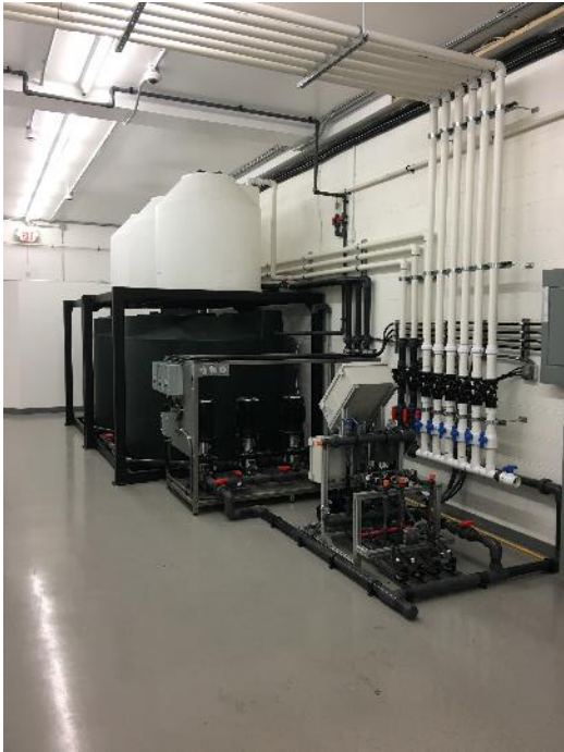
Automated Irrigation System
