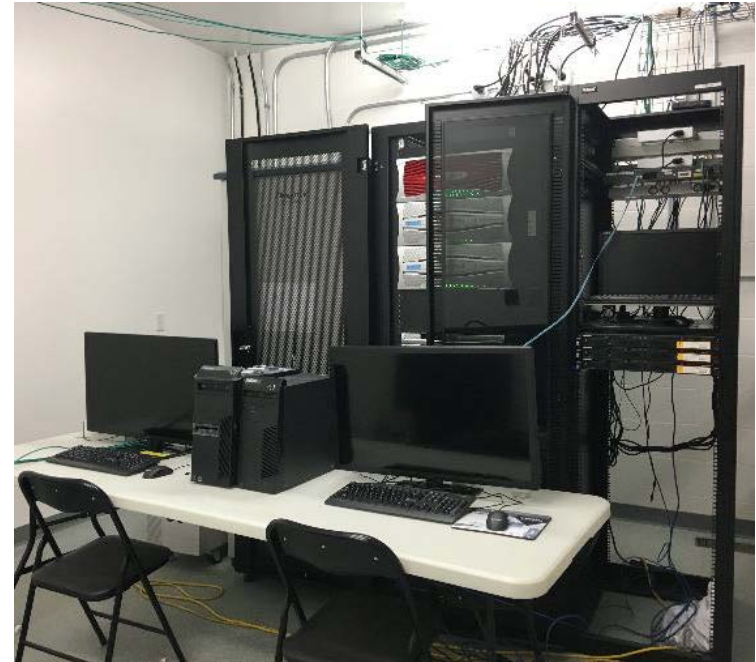
Servers for Security Surveillance System
