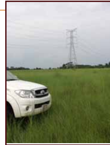
High voltage power lines
