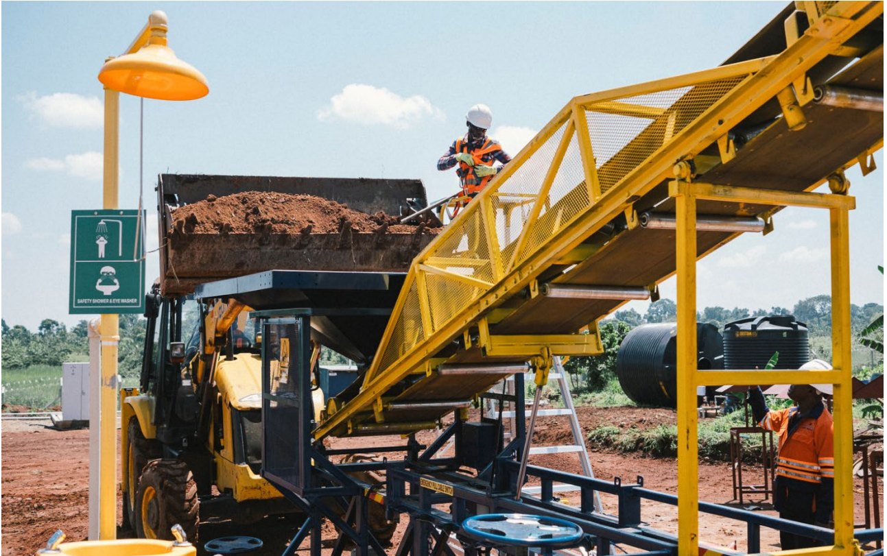
Figure 1: Ore loading of agglomerator feed conveyor.
