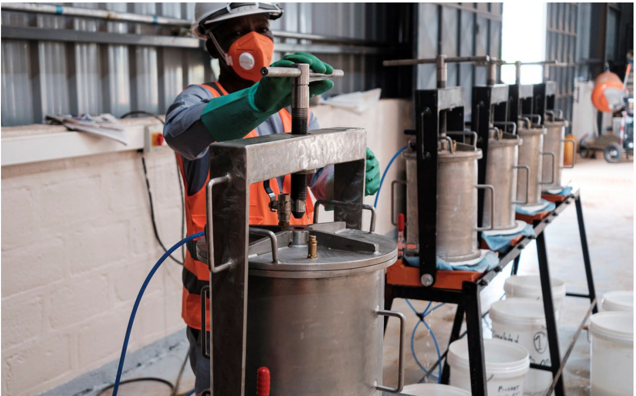
Figure 6: Commissioning filter presses for MREC precipitate filtration.
