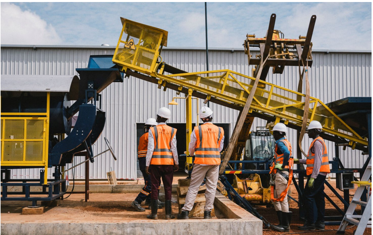
Figure 2: Conveyor to load agglomerator and desorption cribs.
