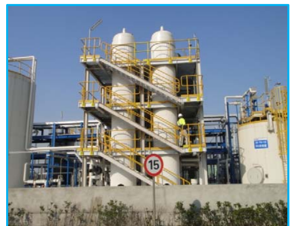
Ion exchange units performing well
