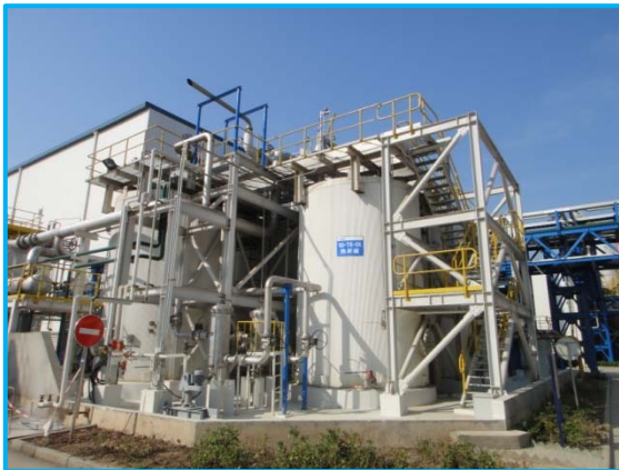
Purification plant in operation
