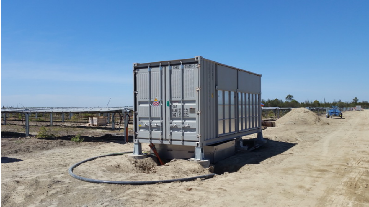
Figure 4: Inverter module installed.
