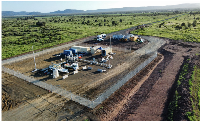
Figure 1: Completed CNG Facility including all weather access road (top of photo) leading to Carnarvon Highway.
