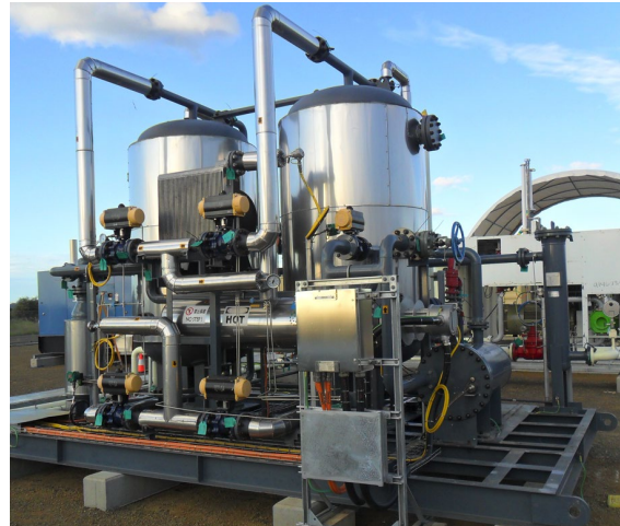
Figure 4: Commissioned dehydrator package, capable of reducing moisture content to less than 35mg/sm 3
