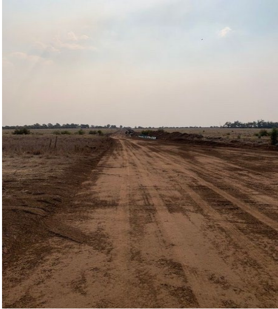
Figure 1: Enabling civil works – construction of tracks, laydown area and longer term access road
