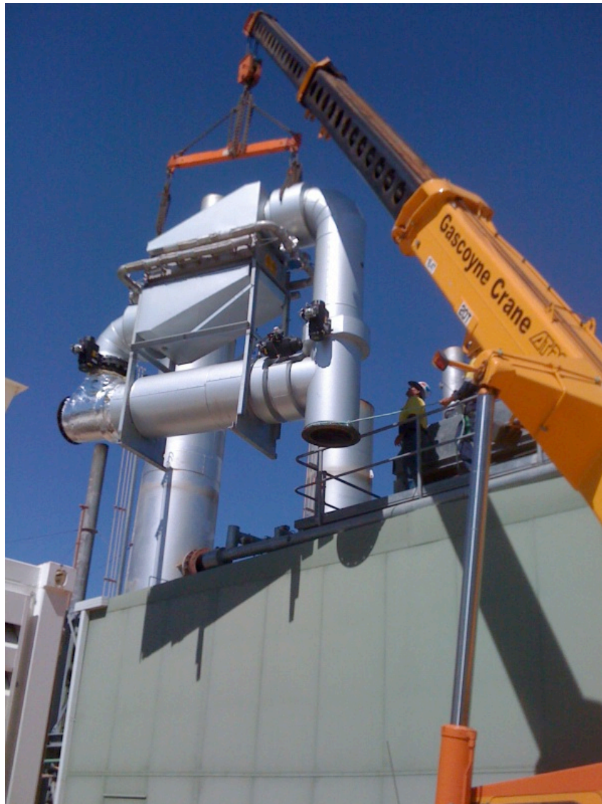
Figure 1–The first heat recovery unit (HRU) is installed in Carnarvon
