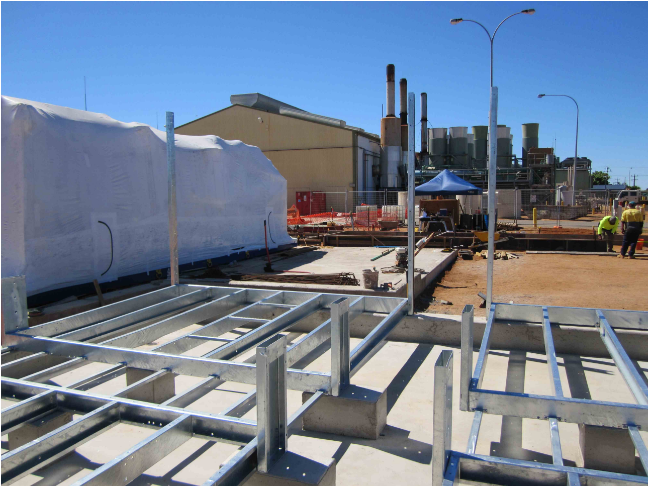
Figure 2—Cooling tower assembly with the Opcon Powerbox and the pumps' concrete base in the background
