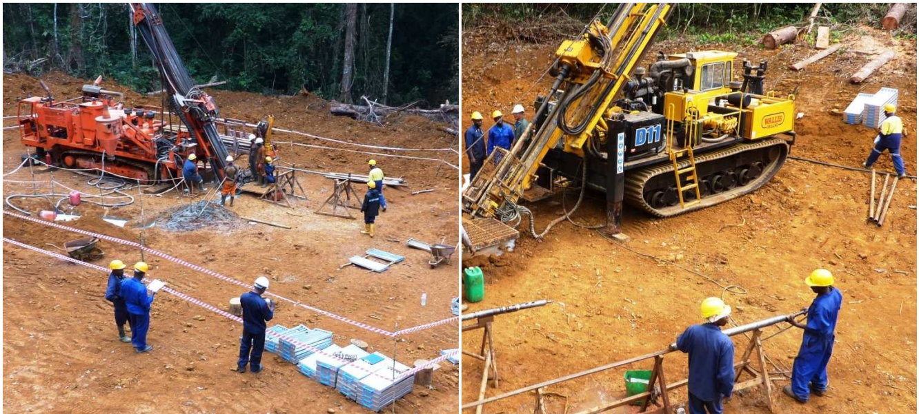
Figures 3 & 4: Partners Drilling and Wallis Drilling – diamond drill rigs in action at Makengui
