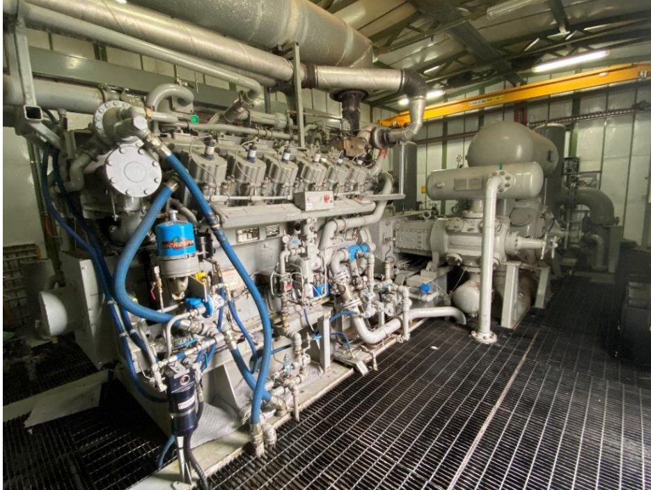
One of the compressor engines at the Rosalind Park Gas Plant
