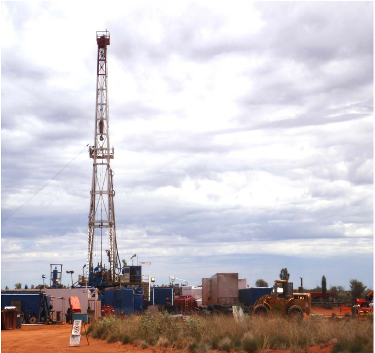
Drill rig in operation at Surprise-1 Re-entry Horizontal well on EP115 in Northern Territory
