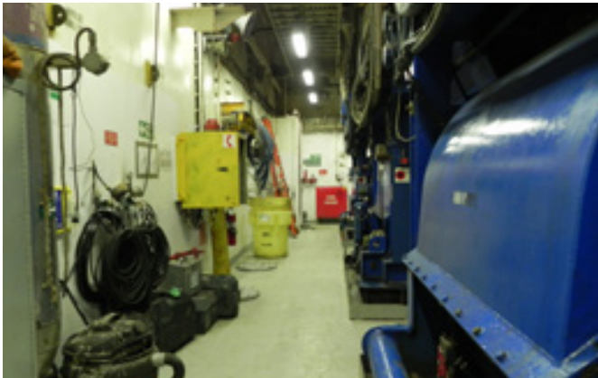
MAIN MUD PUMPS ON THE LOWER DECK
