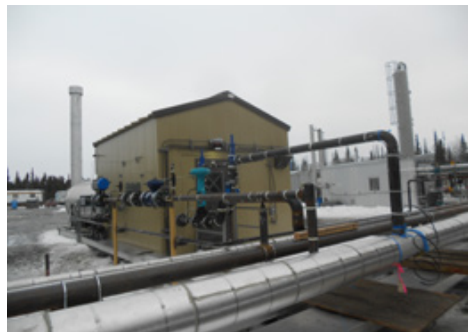
KENAI LOOP PERMANENT PRODUCTION FACILITIES
