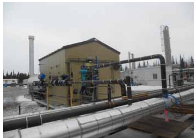
KENAI LOOP PERMANENT PRODUCTION FACILITIES
