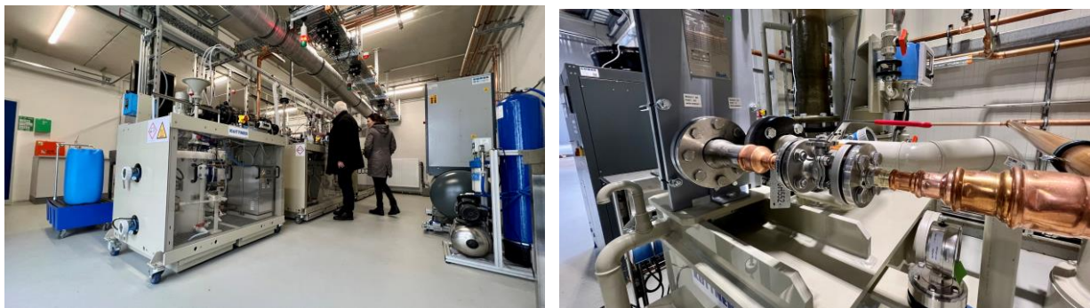
Figure 8 - Pilot Plant in Dock3 facility, Schwarze Pumpe Industrial Park, Saxony, Germany
