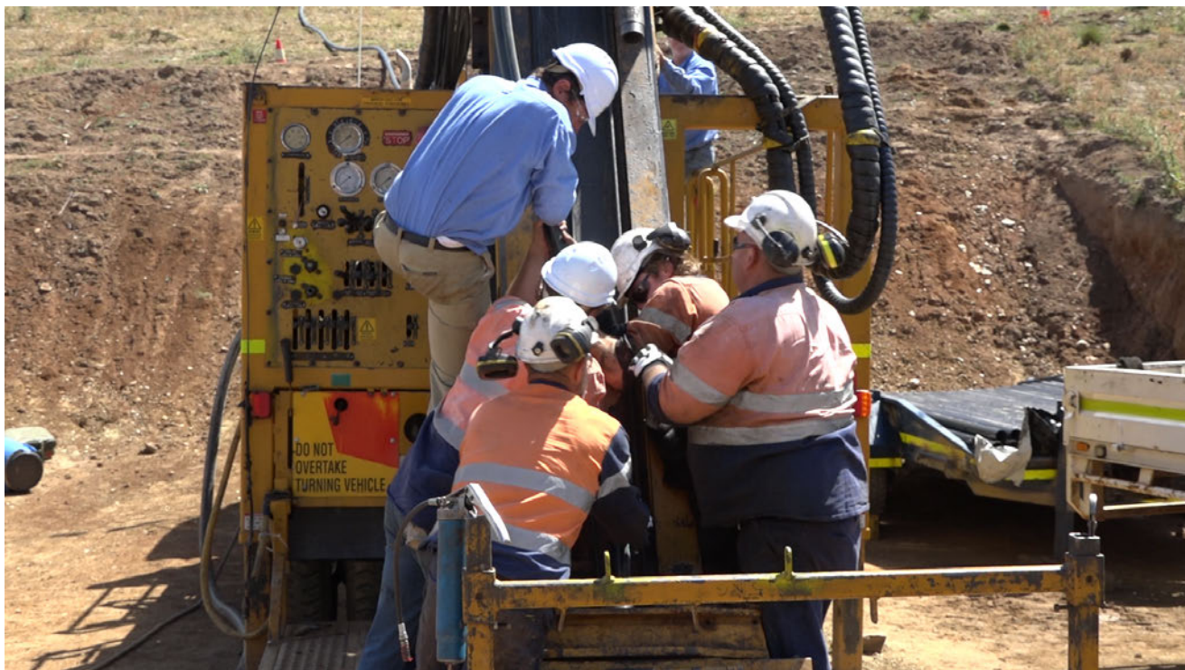
Figure 4 - Drilling crew, site manager and geologist effort in casing the final stages of Hole #2
