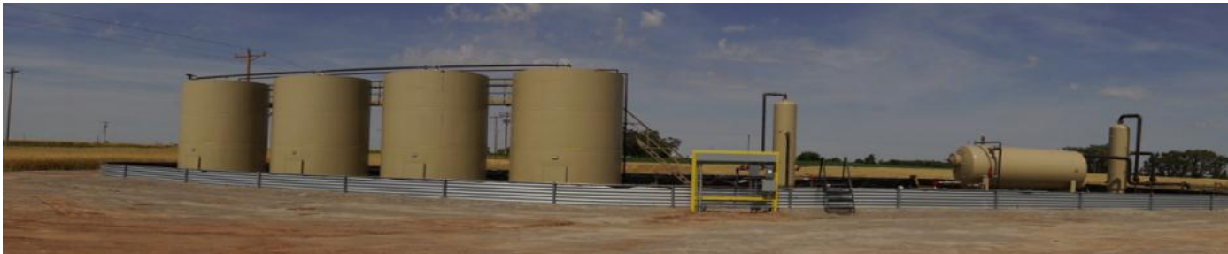
Balder #1 Tank Battery
