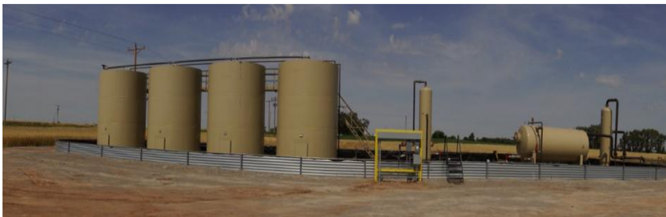
Figure 3: Balder #1 Tank Battery
