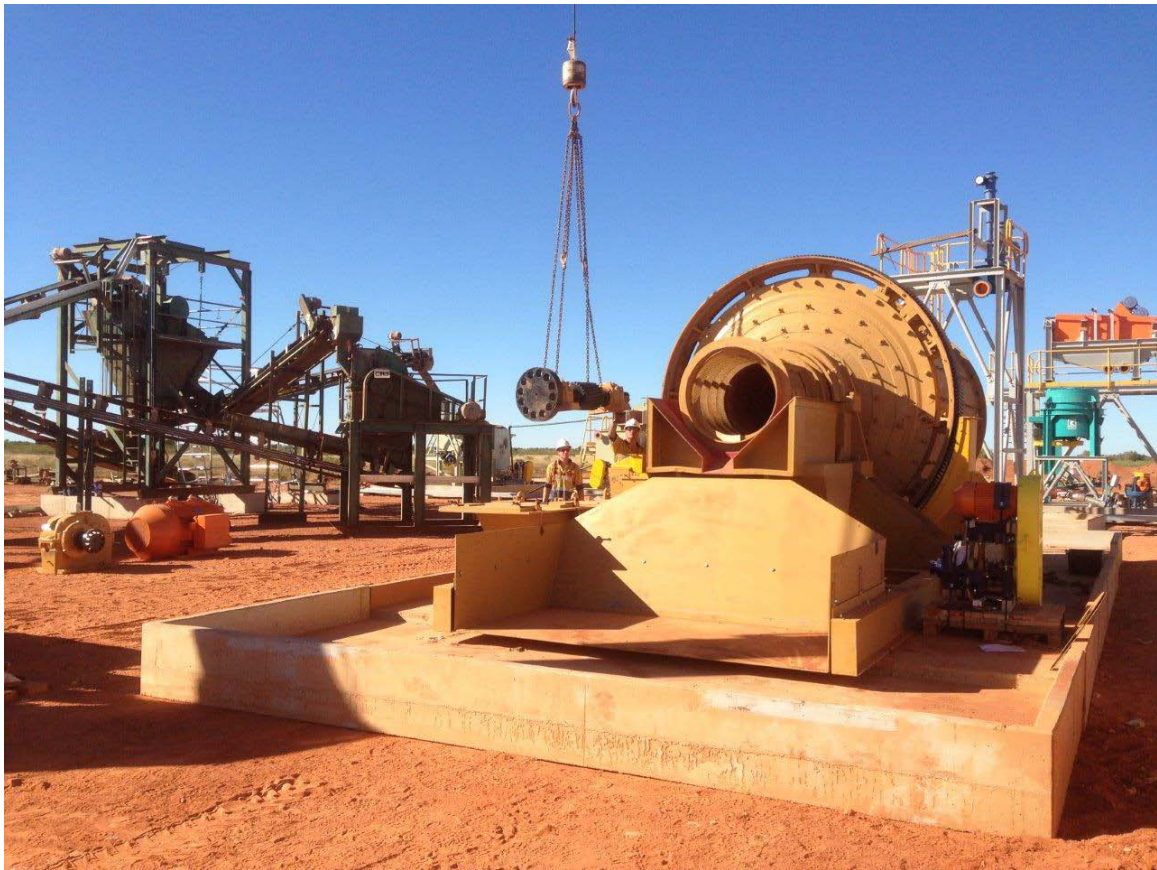
Figure 7. Ball mill in place. Crushing plant to the left installed and tested; photo taken 4 days ago. Cyclone tower, screen decks and knelson concentrator installed (at the back to the right).
