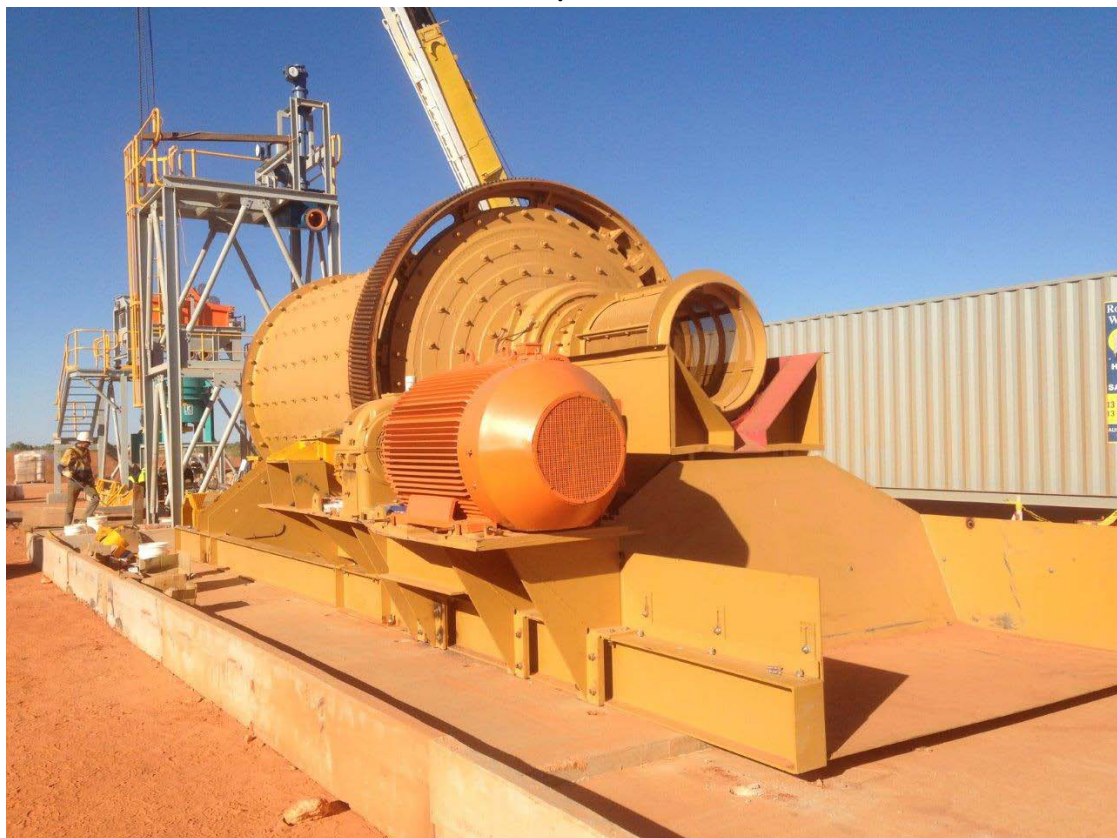
Figure 8. Ball mill in place with motors attached; with cyclone tower and Knelson concentrator (left back). To the right is the containerised concentrate upgrade / gold tabling room. Photo taken 2 days ago.
