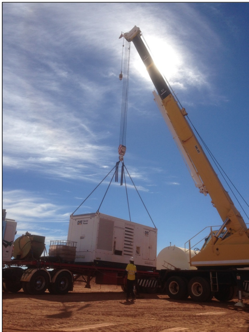
Figure 1. Generator Set being loaded into position with fuel tanks in the background to the right.
