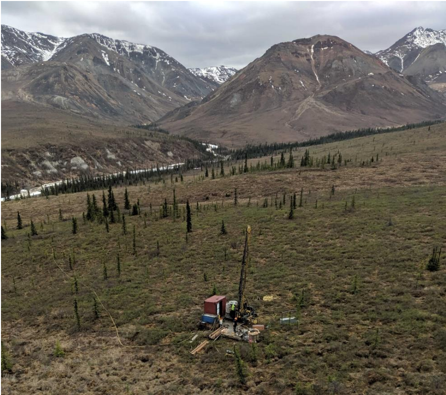
Figure 2: Diamond drill rig set-up 2km west of the WTF deposit, looking south towards Red Mountain.
