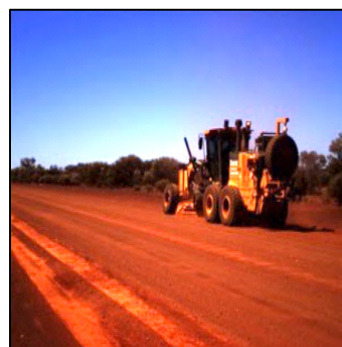
STATION ROAD 85KM
