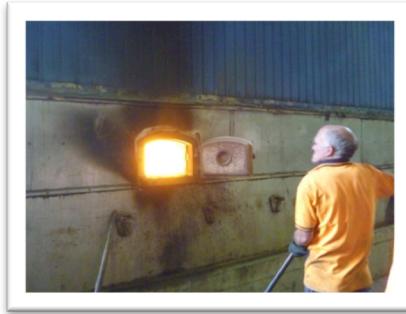
Coldry performed well in the furnace
