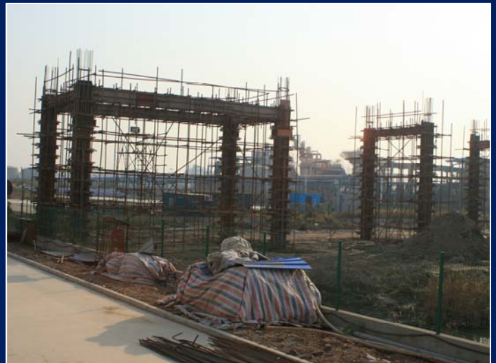
Pipework support structures
